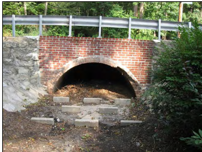
This arched culvert, OT-01, discharges to the box culvert that conveys Cold Spring Brook beneath Harbor Road.
